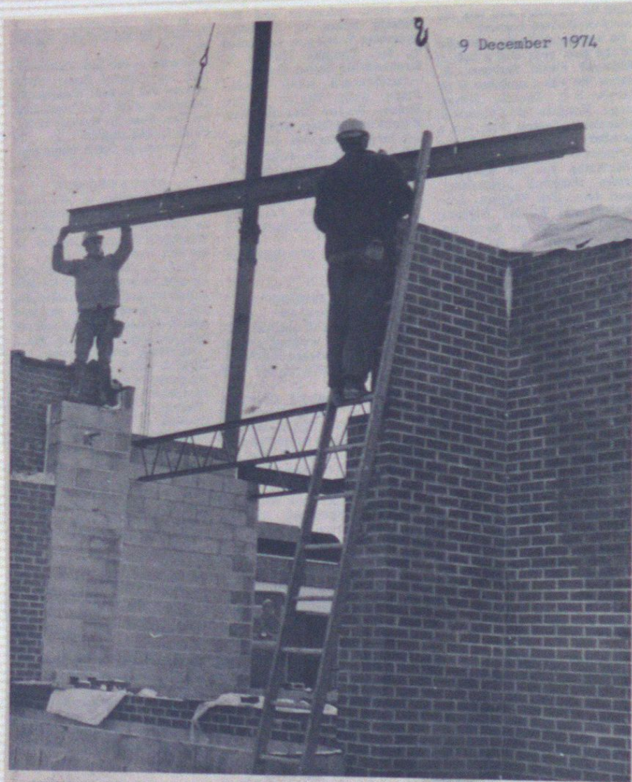
8 9 December 1974 A major step in the construction of the new Tillsonburg Public Library was made on Friday, with the installation of the steel beams. The construction, by Gilvesy Construction of Tillsonburg, is proceeding according to schedule and the new library facility should be opened some time in late Spring of 1975.
